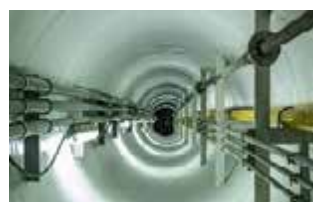
Low pressure pipelines
